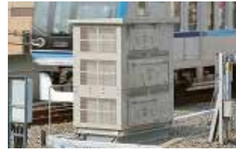
Station auxiliary power supply unit
