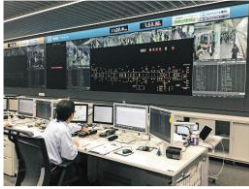
Integrated Control Center (OCC)
