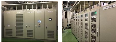
Stationary energy storage system
