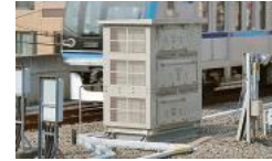
Station auxiliary power supply unit
