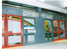
Platform screen doors
