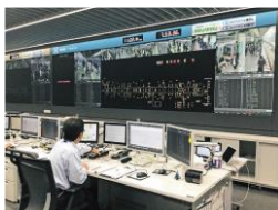
Integrated Control Center (OCC)
