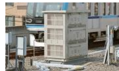
Station auxiliary power supply unit
