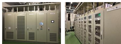
Stationary energy storage system
