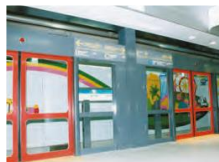
Platform screen doors
