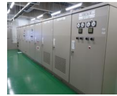
Power transmission and distribution
