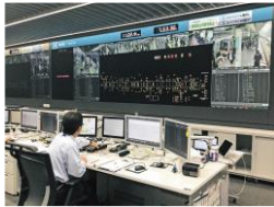
Integrated Control Center (OCC)
