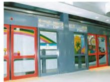
Platform screen doors
