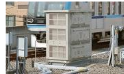
Station auxiliary power supply unit
