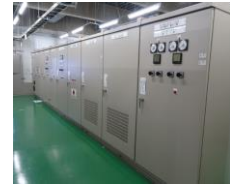
Power transmission and distribution
