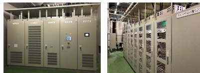
Stationary energy storage system
