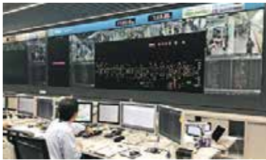
Integrated Control Center (OCC)
