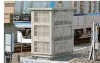
Station auxiliary power supply unit
